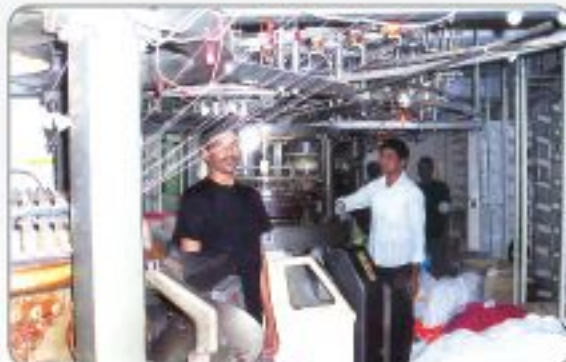
Inside view of Florescent Apparels Ltd. financed by SBL, Principal Branch, Dhaka.
